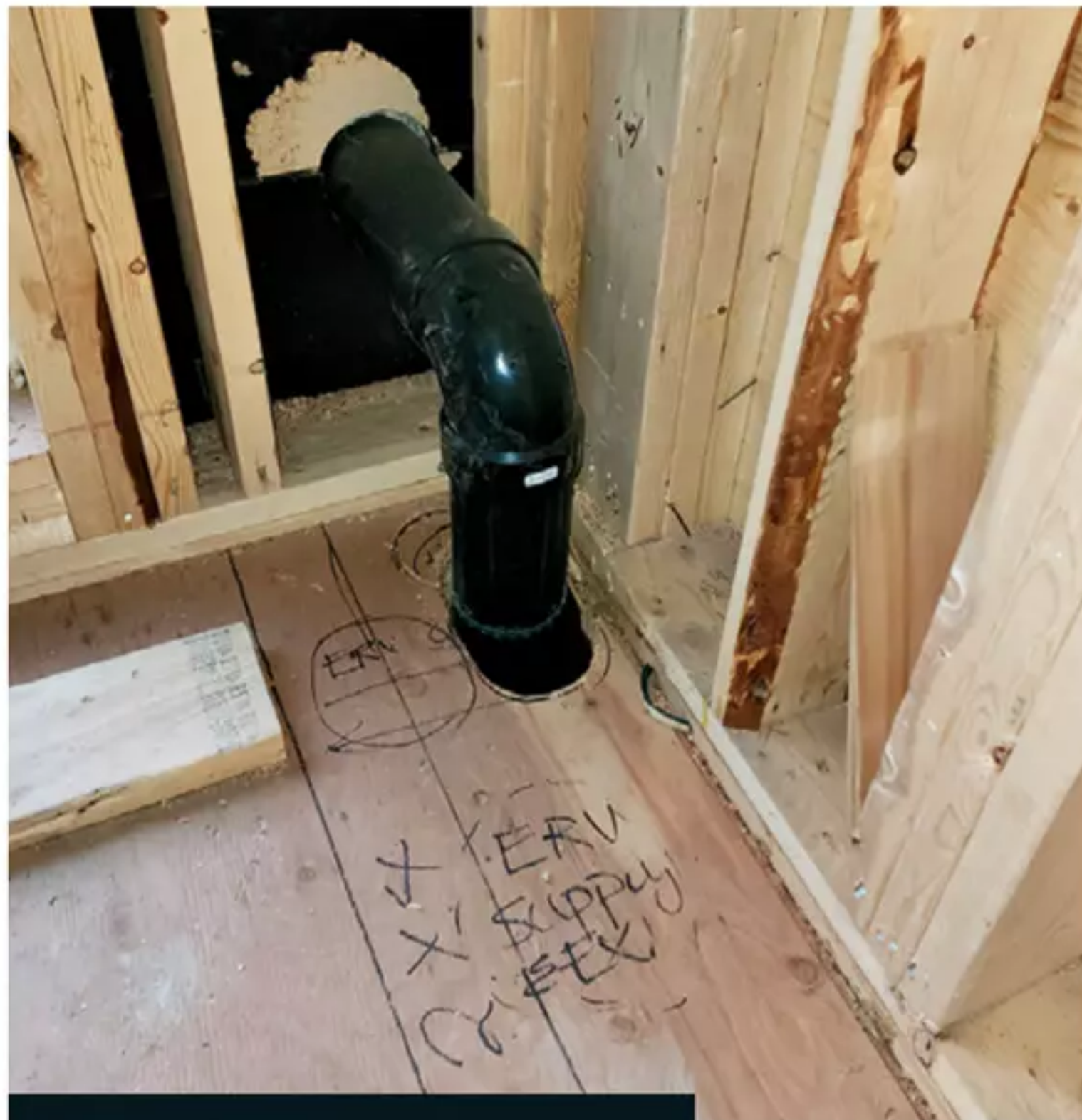
Outlet for sub-slab radon venting system.
